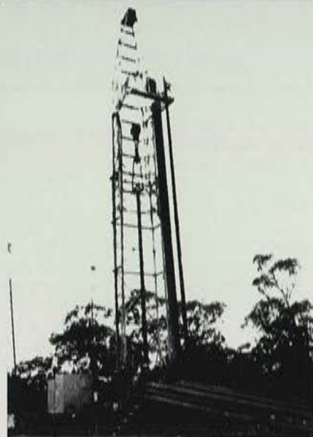
Cardwell HL drilling 711 mm hole to 477 m using air hammer techniques. Probably the largest and deepest hole so drilled in Australia. Running drill pipe to bottom, Tower Colliery.
