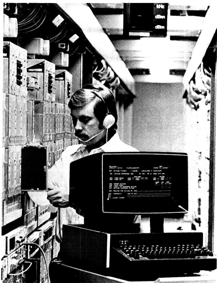
Fig. 8—Terminal Equipment Center (TEC).
