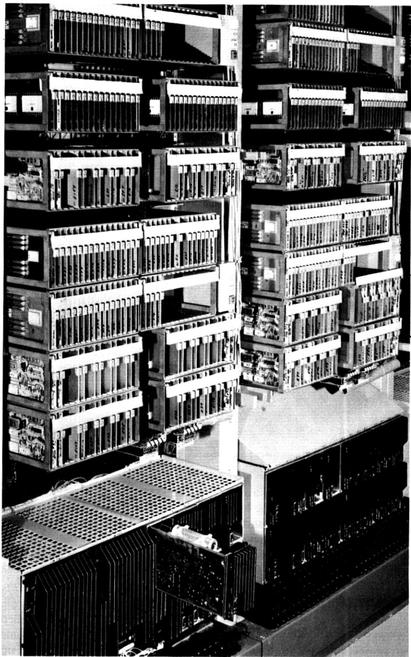
Fig. 6—No. 4 ESS frames with power shelves. One 3-V, 8-A converter is shown partially withdrawn at bottom.
