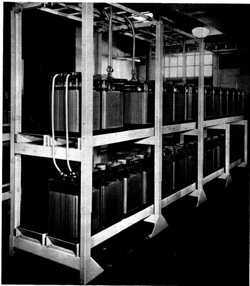
Fig. 1—Battery rack for normal service.
