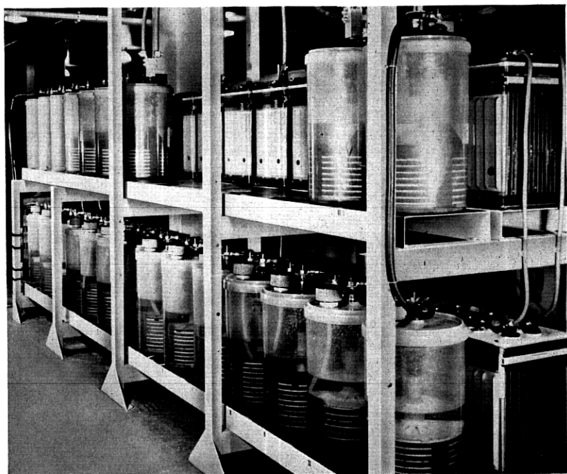
Fig. 12—Trial installation at Murray Hill, New Jersey Bell Telephone Co. Central Office.
