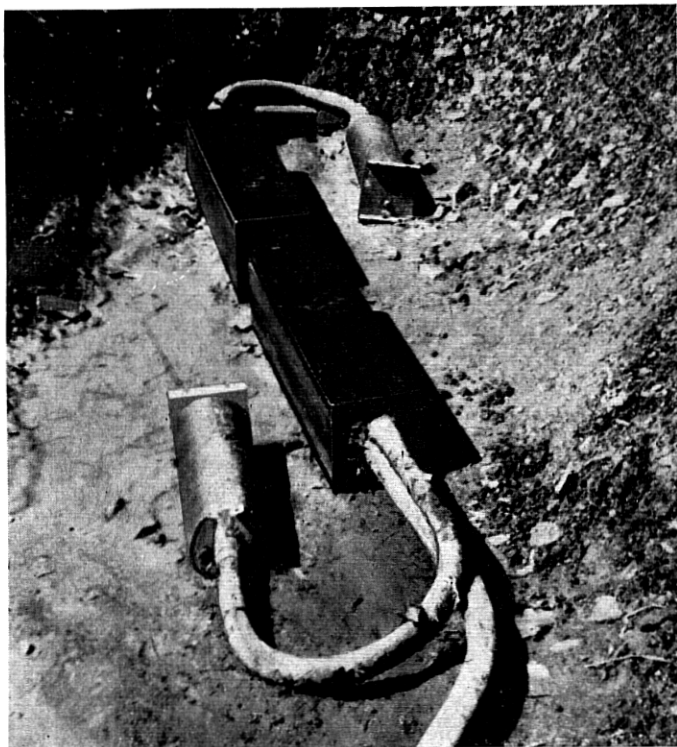
Fig. 29—Buried coaxial cable installation of voice-frequency loading on outer layer quads. View of installation after completion of the splicing work, and prior to filling in the excavation. The loading coils are potted in two tubular, thin steel, cases. Each of black boxes near center covers a cable splice, and furnishes protection against mechanical injury. At each splice, connections are made to the stub cable conductors of a single loading coil case. Splicing difficulties prevent all of the connections from being concentrated at a single cable splice.
