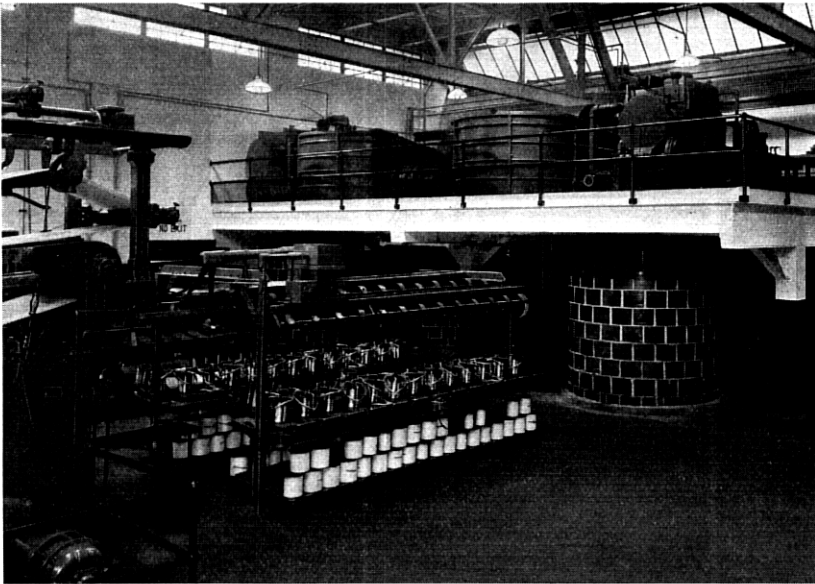
Fig. 3—Wire supply and pulp preparation equipment.
