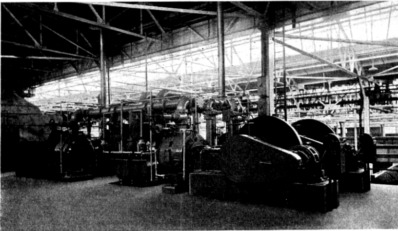
Fig. 16—Auxiliary equipment for vacuum driers.
