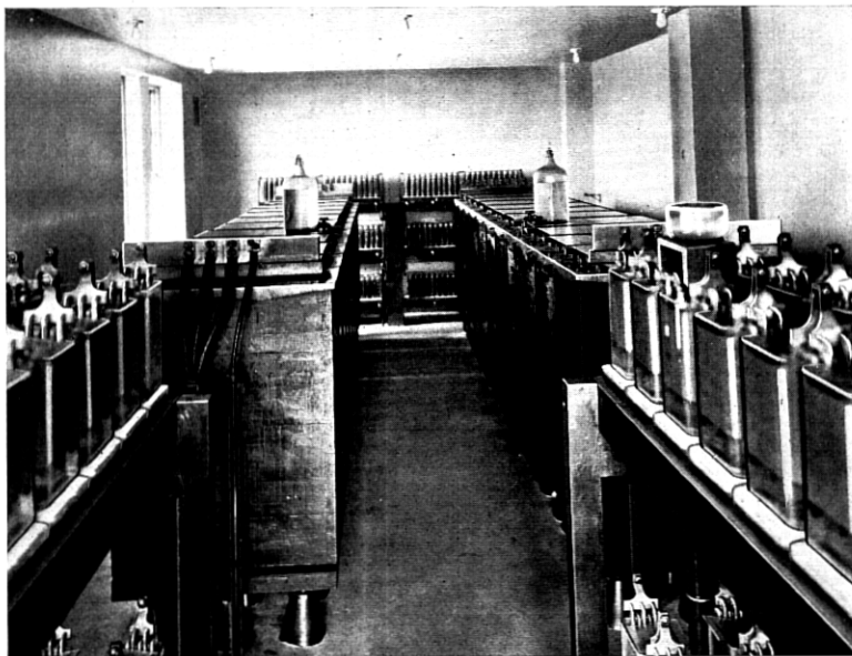
Fig. 9—Typical Storage Battery Room for Cable Repeater Station
